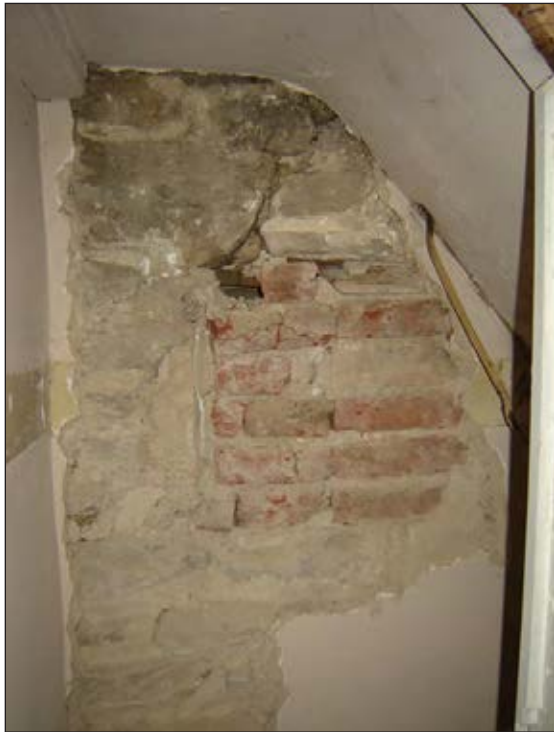
Figure 4 A bricked up window or vent on the third floor of the old west wall of Sellers Hall. The window was likely covered when a roof for building A was built.
