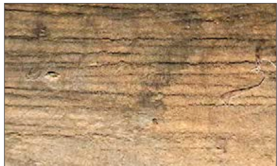
Figure 2 Pit saw marks, 2010.
