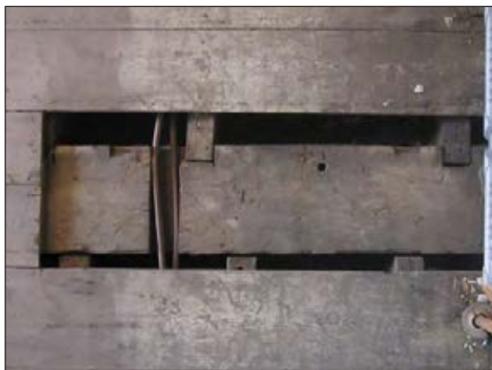
Figure 5 Chimney girt in room 202, 2010.
