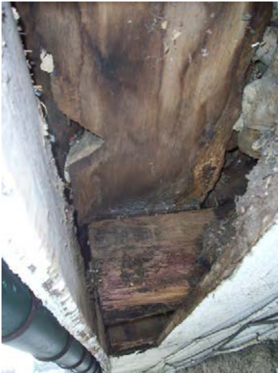
Figures 10 & 11 Images of the original cornice. The stone of the knee wall can be seen through gaps and notches in the board.
