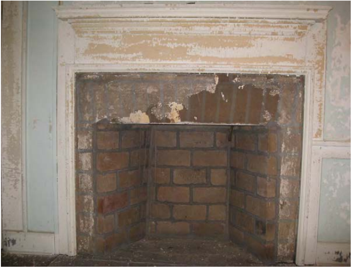
Figure 12 Image of a fireplace highlighting the multiple campaigns of faux-brick finish.
