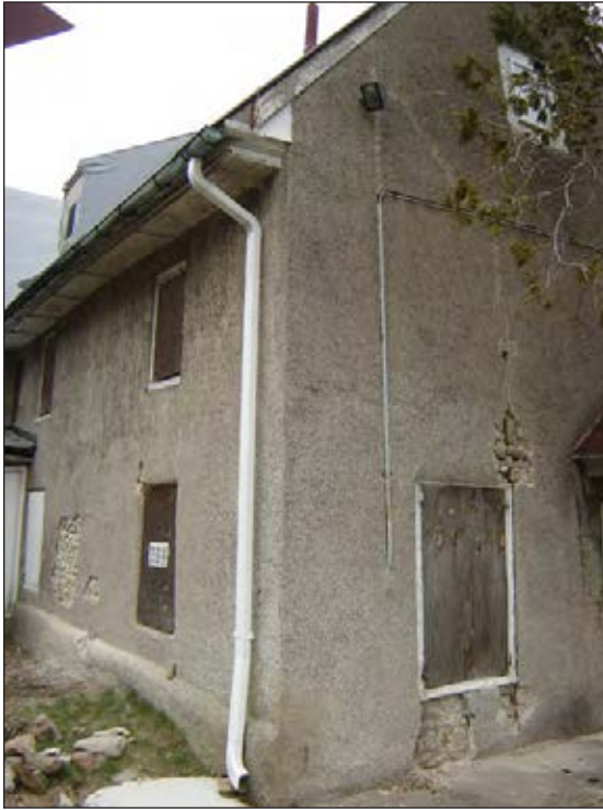
Figure 5 2011 image of the northwest corner of the western addition – a crack in the stucco of the west face represents a seam between buildings A and B.
